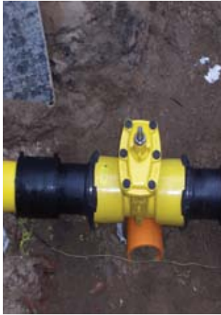
Gas network Bialystok, Poland VAG EKO plus Gate Valves with welding ends
